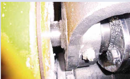
Discharging leaks when utilizing compression packings increases the risk of dust explosion
